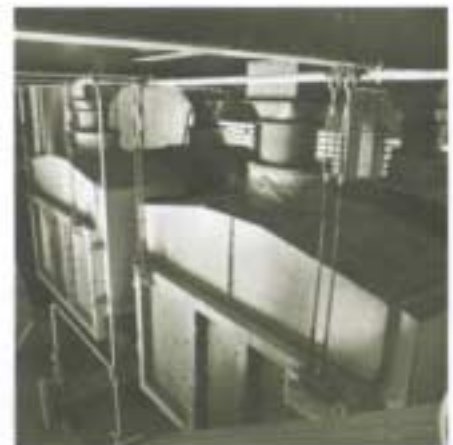
Cable-suspended ROTEX and MEGATEX Screeners minimize transmission of motion to adjacent structures. Two Model M4260 MEGATEX are shown.
